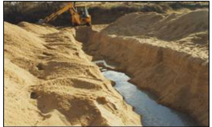
(Above) Shashe sand river trenched at Gulubane, N.E. Botswana: note shallow water table
