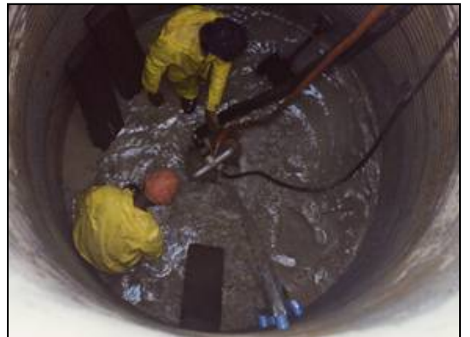
(Above) Flow of about 4 l s -1 from sand river through laterals into Gulubane collector well
