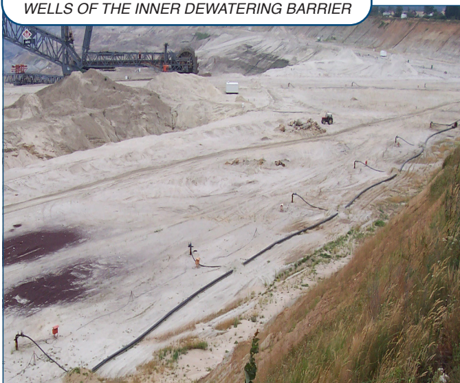
BELCHATÓW LIGNITE MINE — POLAND WELLS OF THE INNER DEWATERING BARRIER
